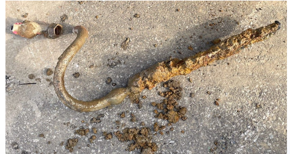
Example lead gooseneck and corroded lead service line. Erie City Water Authority – City of Erie, Erie County
